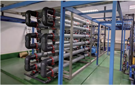
480m³/d Tubular Membrane Treatment System for Chip Grinding Wastewater
