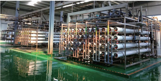
3200m³/d Landfill Leachate and 640 m³/d Concentrate Nanofiltration Full-Scale Treatment System
