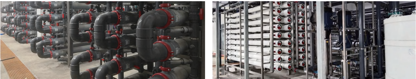
150m³/h Mine Water Zero Liquid Discharge Treatment System for a Coal Mine in China National Coal Group
