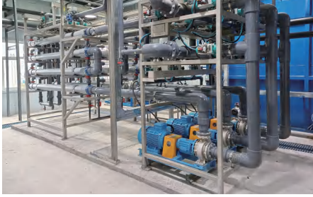
40m³/h Coking RO Brine Silica Removal System
