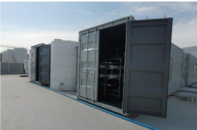
▲ 200kg/h Industrial Waste Salt Resource Utilization Project
