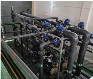
▲ 500m³/d Oilfield Produced Water Oil Removal Project
