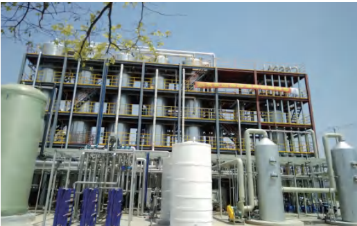
2000 m³/d Ammonia Stripping Project for Ammonium Bicarbonate Preparation in Shanghai
