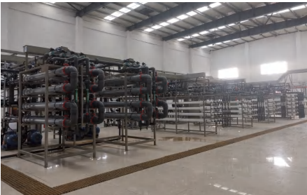
▲ 1350m³/d Iron-contaminated Wastewater Heavy Metal and Hardness Removal Project for a Steel Plant
