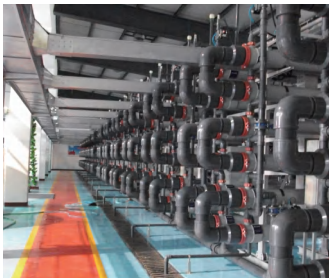
▲ 10000m³/d PetroChina Oilfield Produced Water Oil, Impurity Removal and Demineralization Project
