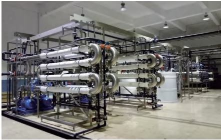
425m³/d External MBR System for Landfill Leachate
