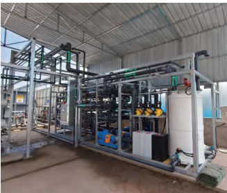
▲ 200m³/d Oil and Gas Mud Filtration Oil Removal System
