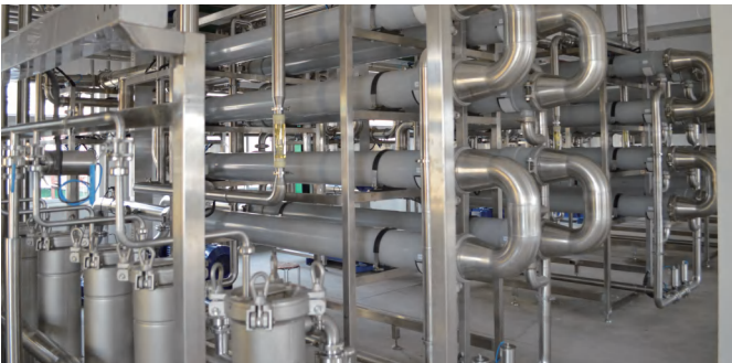
▲ Membrane separation and purification equipment for L-Alanine
