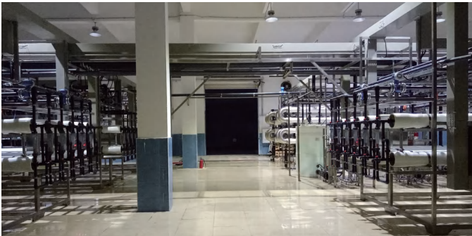
425m³/d Leachate and 300 m³/d Leachate Concentrate Nanofiltration Full-Scale Treatment System
