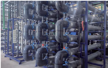
▲ 50m³/h Phosphoric Acid Iron Washing Water Clarification and Heavy Metal Removal System for a New Energy Company
