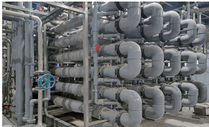
▲ 60 m³/h Fructose Saccharification Clarification Equipment for a corn processing company in Northeast China
