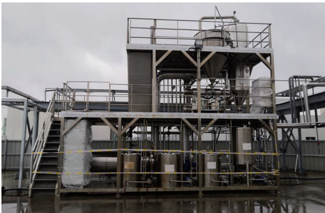
▲ 50,000 tons/year Fly Ash Washing Wastewater Resource Utilization Project
